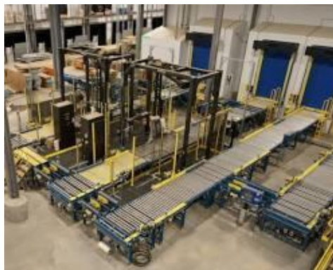
Chain Conveyor in a Cold Storage
