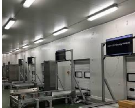
Roller Conveyor in a Cold Storage
